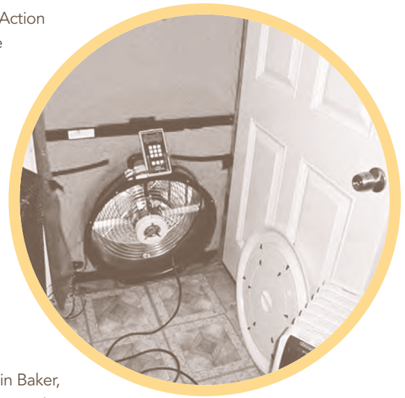
Prior to weatherizing a home, the Northeast Florida Community Action Agency performs a "blower door" test to locate where a home is losing air. Contractors then seal off gaps and cracks in a home to stop unnecessary energy loss.
